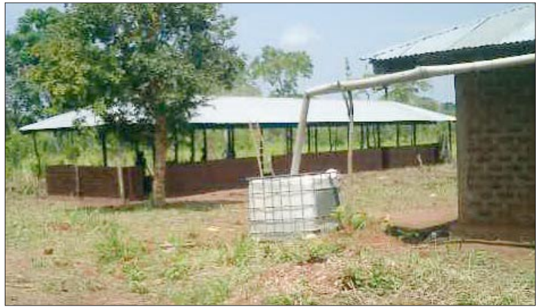
In a short time they put up the roof and raised half of the wall.
